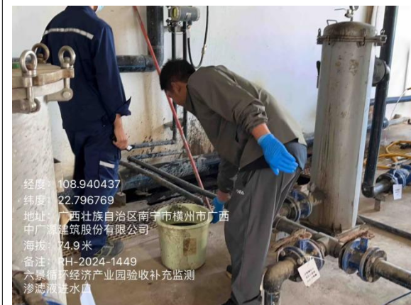
渗滤液进口采样
